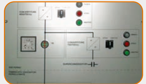
DC/DC converter panel
